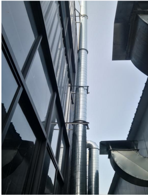
15m高排气筒
